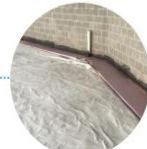
15 Perimeter Foam and Expansion Joint Installed by Concrete Contractor Prior to Pouring Concrete Floor Slab
